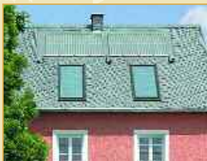
Neatly integrated in-roof mounted TUBO modules - Germany
