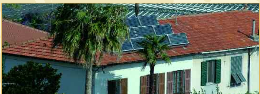
Upright mounting of TUBO 12 CPC collectors on low pitch roof - Southern Europe
