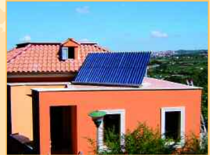
6 TUBO modules on posts, Italy
