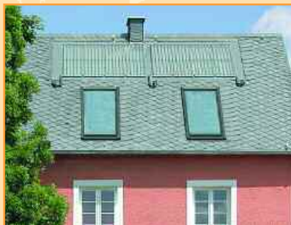
Hardly visibly in-roof mounted TUBO modules, Germany
