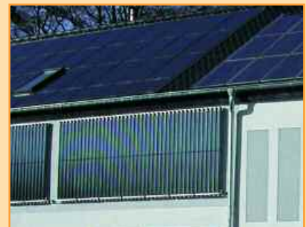
A facade mounting of TUBO, combined with a photovoltaic installation
